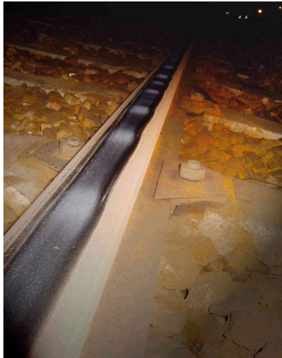
Figure 1. Corrugation on the line A of the Paris RER network between Fontenay-aux-Roses and Robinson stations.
