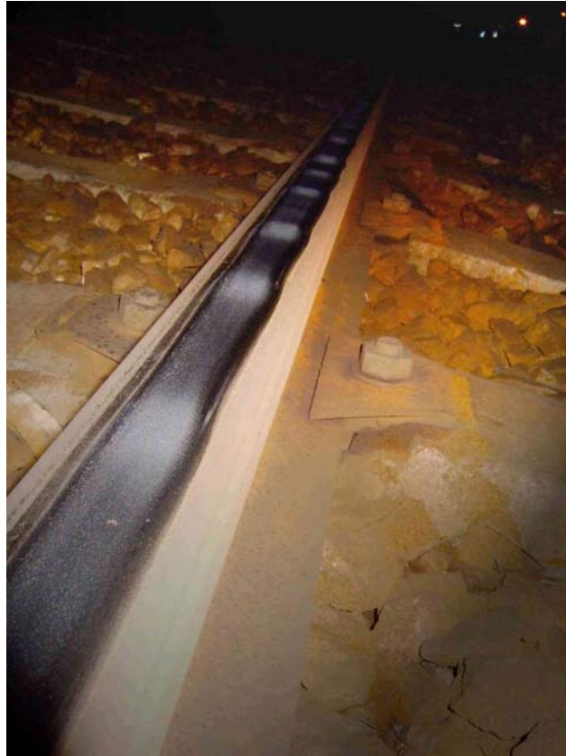
Figure 1: Corrugation on the line A of the Paris RER network between Fontenay-aux-Roses and Robinson stations.
